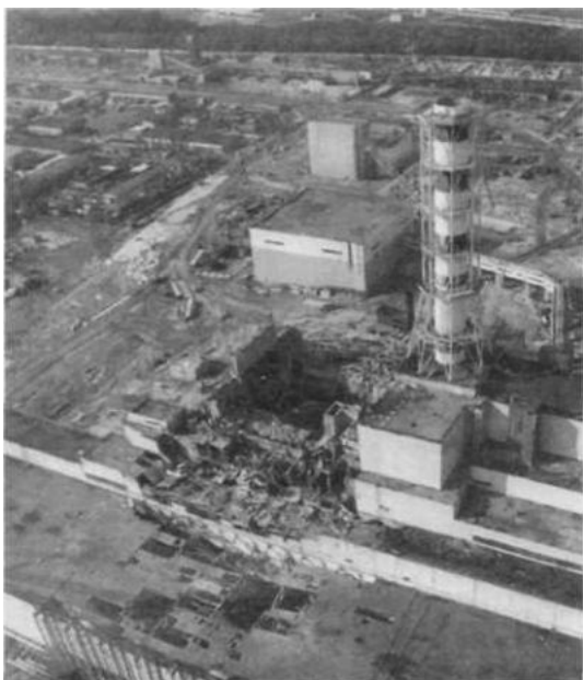
Chernobyl reactor 4 after the tragedy, showing the extensive damage to the main reactor hall
